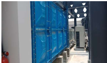
Gambar 15. GWT ( Ground Water Tank ) Bio Septic Tank
