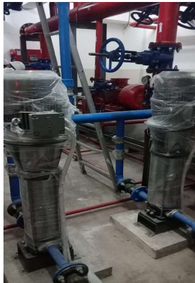
Gambar 17b. Jockey Pump Hydrant (Sumber PT. JAGA CITRA INTI)
