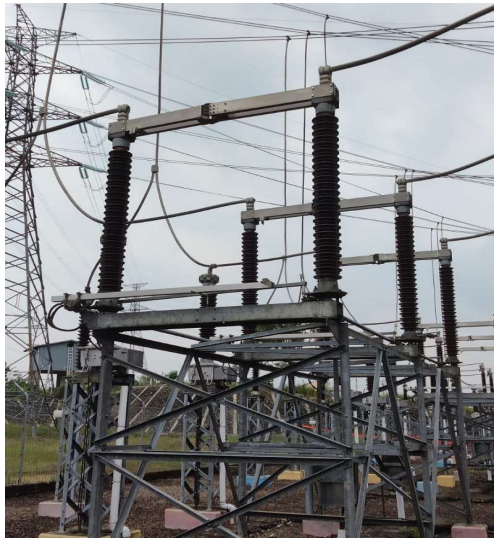
Gambar 1. Disconeccting Switch (DS)
