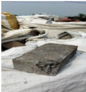
Gambar .6 Defect Paving Gupil
