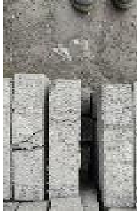
Gambar .4 Defect Paving Retak
