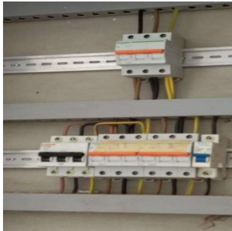
Gambar 4. Panel Utama PT. Multi Group Holding Company
